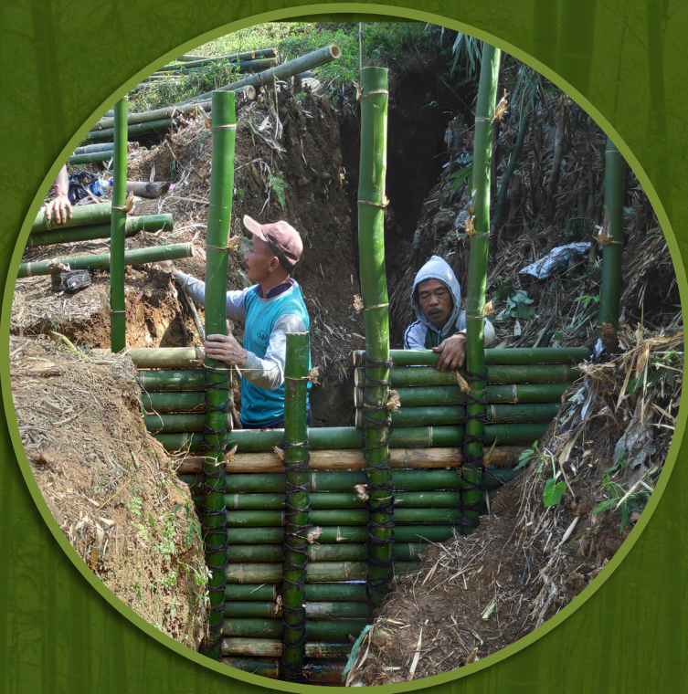
Bamboo gully plugs to prevent erosion and sedimentation, and to control gully development. Photo credit: WMTC
