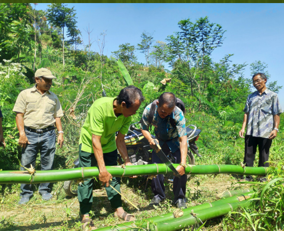
Demonstrating the use of bamboo to control gully erosion. Photo credit: WMTC
