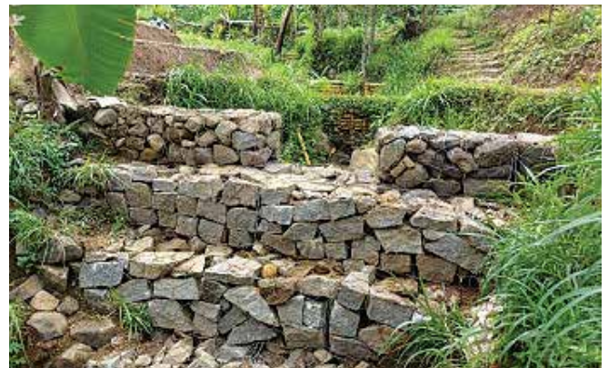
Before and after the construction of a gully plug for controlling water erosion in fields along steep slopes
